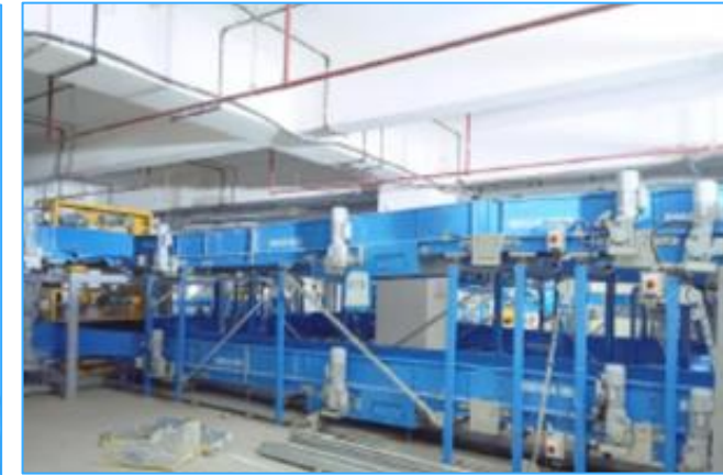
East Processor – Level C
